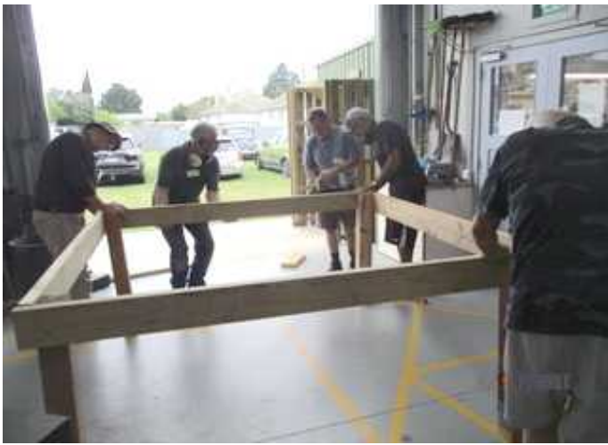
Progress on the chook house. What a difference a couple of weeks makes. The chook house is being built for Marewa school.
